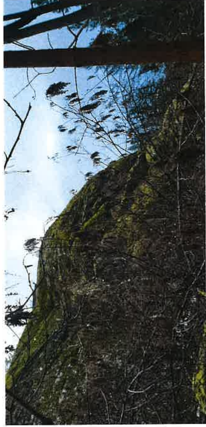
Photo 12 -- Bedrock with Some Loose Rock (WP15)
