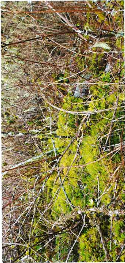
Photo 13 – Moss Covered Rockfall Originating from 10m High Bluff (WP15)
