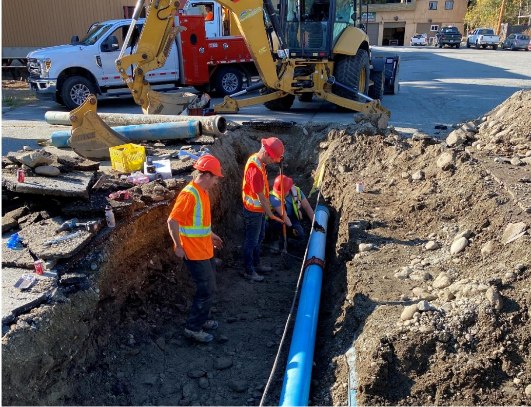
Figure 2 – Watermain break repair on Aster St, October 2022.
