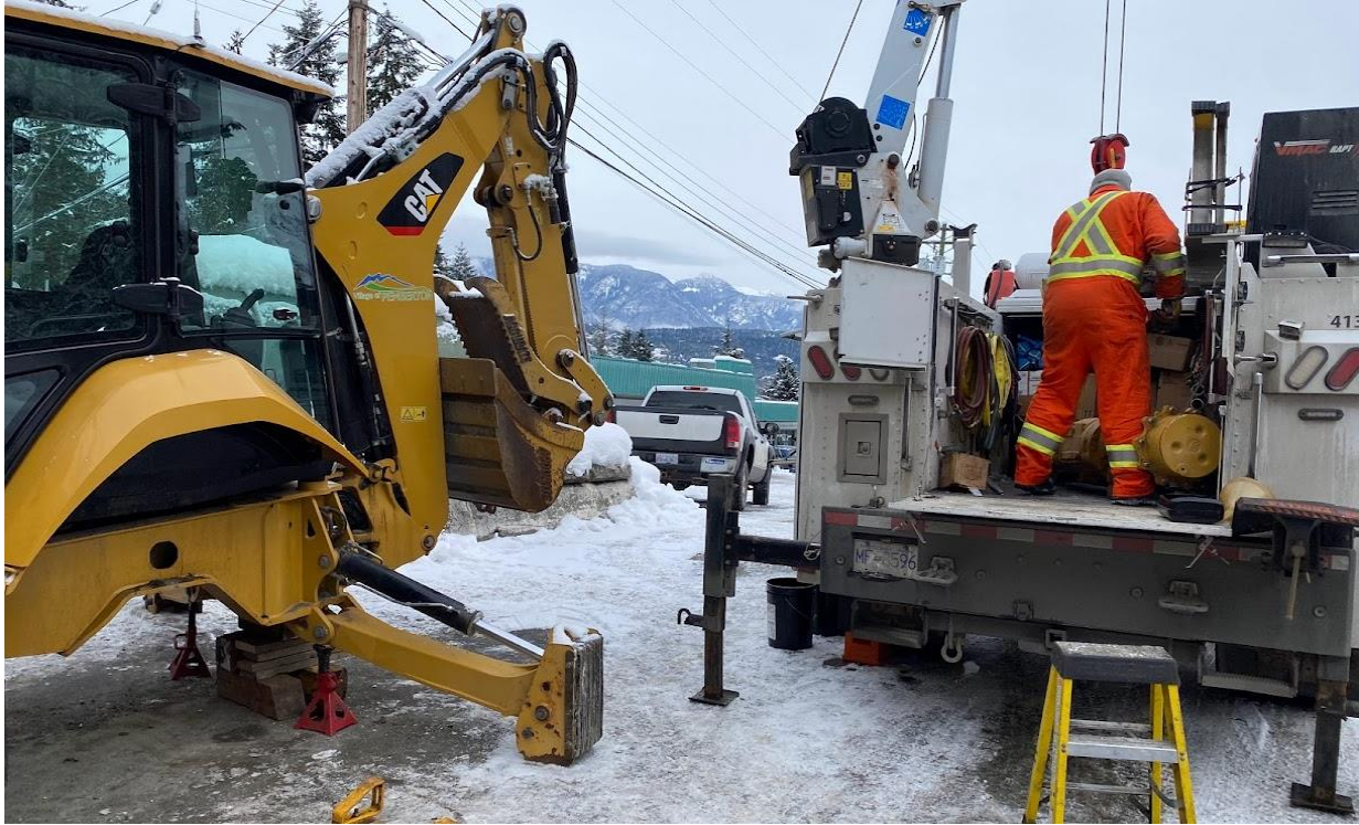
Figure 6 – Hydraulic brake system failure on Backhoe
