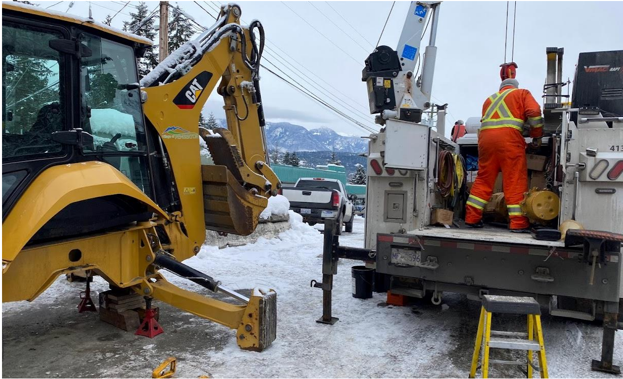
Figure 6 – Hydraulic brake system failure on Backhoe
