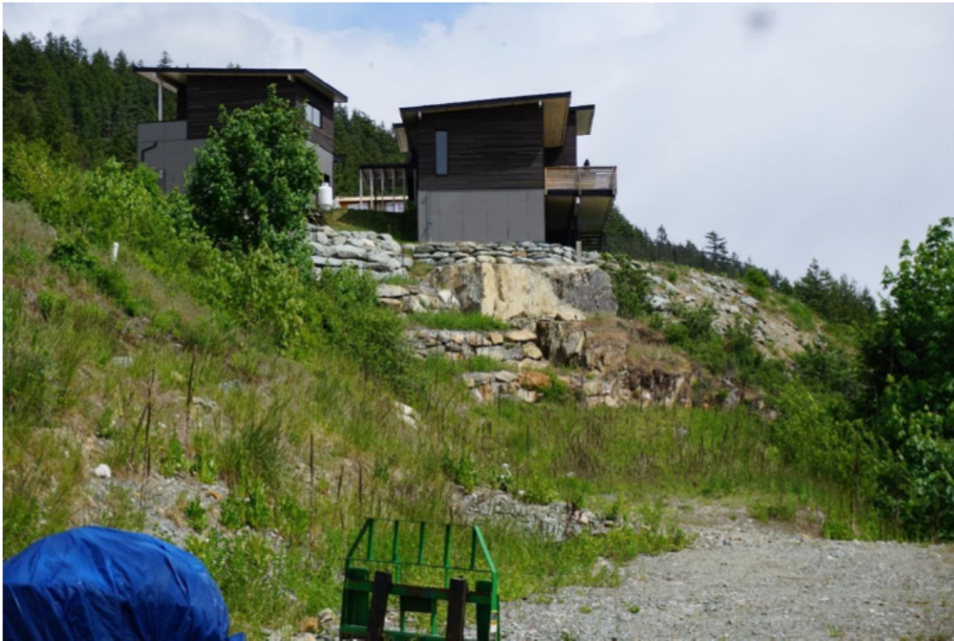
Figure 7 – Local retaining wall example 1 of 6. Example of well executed terraced walls. Location: The Ridge.
