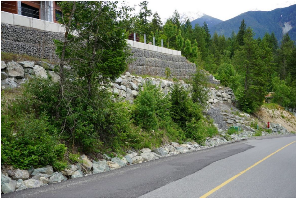
Figure 9 – Local retaining wall example 3 of 6. Example of how each row of gabions step back to easily achieve a 1H:1V slope. Location: main access to The Ridge.
