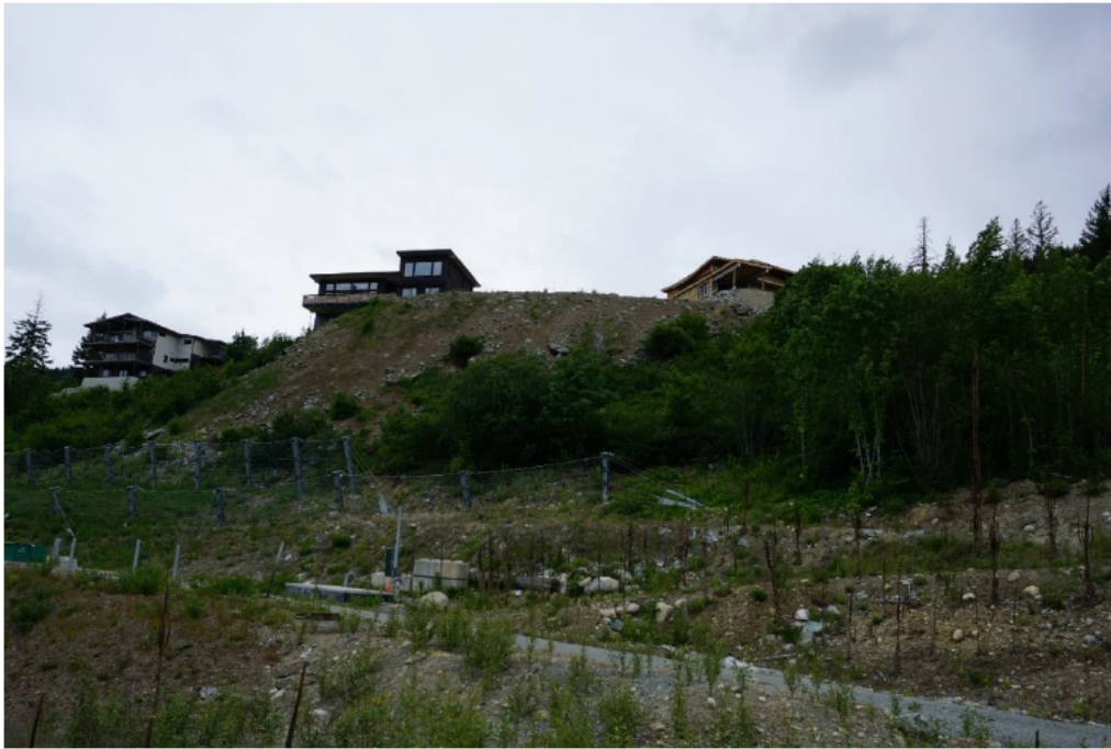
Figure 11 – Local retaining wall example 5 of 6. Example of an unretained slope. Viewed from Sunstone Development.
