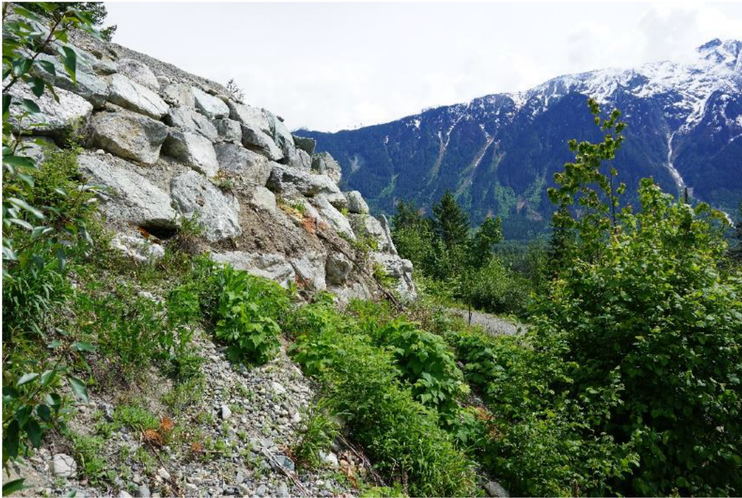
Figure 5 – Current view southwest from within the subject lot, showing extent of neighbouring retaining. This example of existing retaining does not meet current bylaws.
