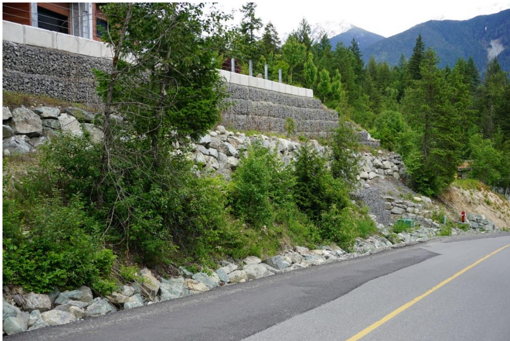
Figure 8 – Local retaining wall example 3 of 6. Example of how each row of gabions step back to easily achieve a 1H:1V slope. Location: main access to The Ridge.
