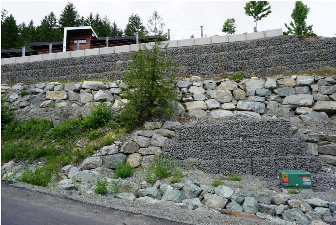
Figure 7 – Local retaining wall example 2 of 6. Walls over height but including terrace for planting. Location: main access to The Ridge.
