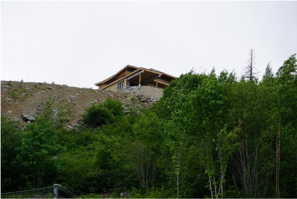
Figure 9 – Local retaining wall example 4 of 6. Example of 1H:1V slope. Although considered acceptable, this solution is not aesthetically pleasing, and prone to erosion. Terraced retaining provides better vegetation cover, less erosion, and a more pleasing appearance. Viewed from Sunstone Development.
