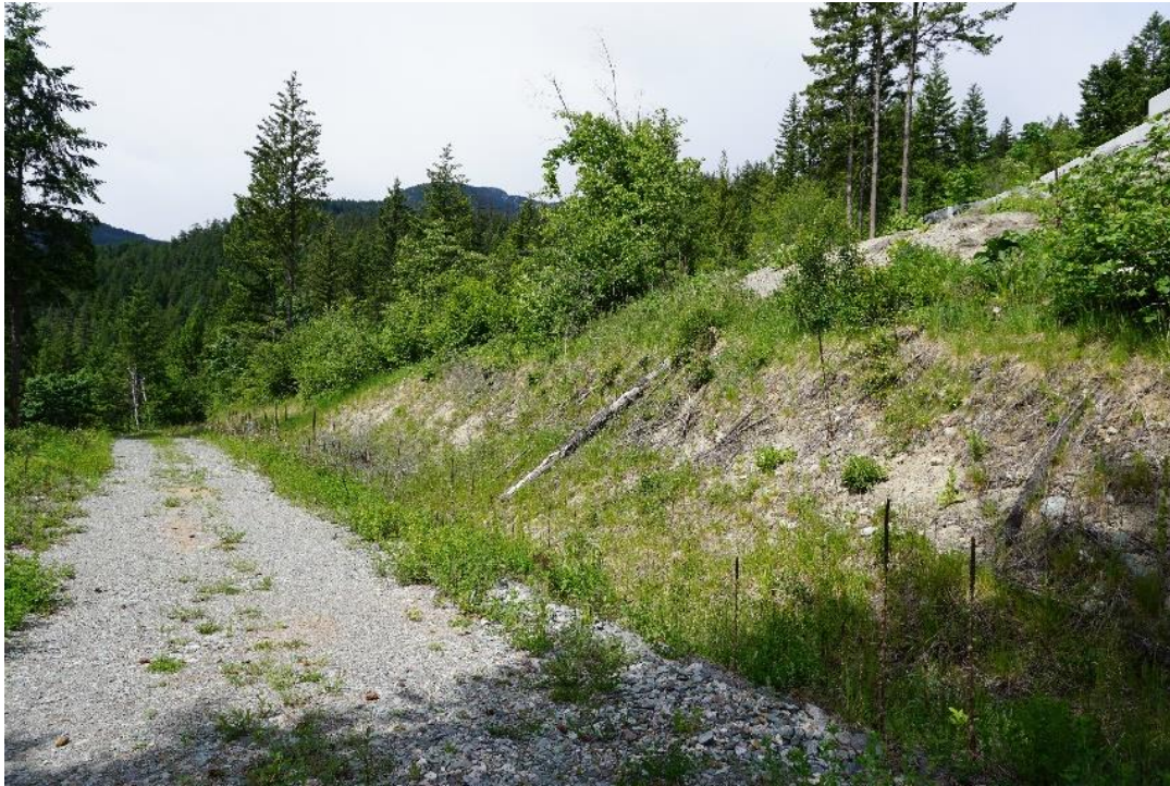
Figure 3 – Current conditions at southeastern corner of the property line looking west. Steep banks and vegetation growth alongside the access road at the rear of the property
