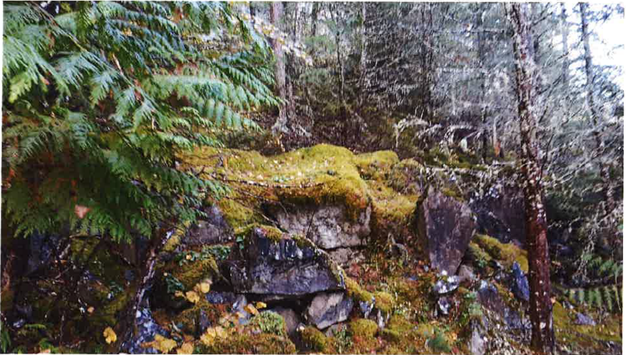
Photograph 15 – Loose Boulders Above Lower Access Road – P15
