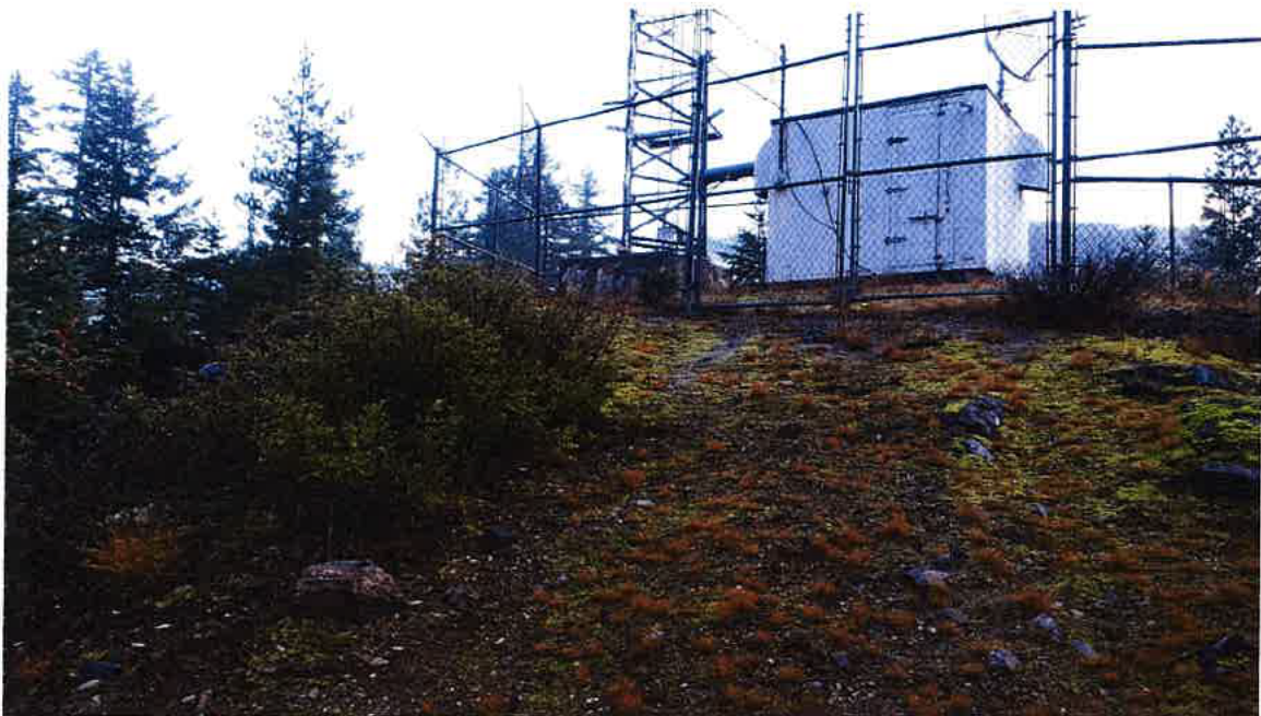
Photograph 2 – Communication Towers – P2
