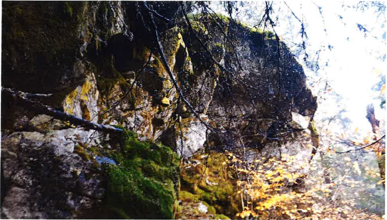
Photograph 3 – Overhanging Bluff, Rockfall Source– P3
