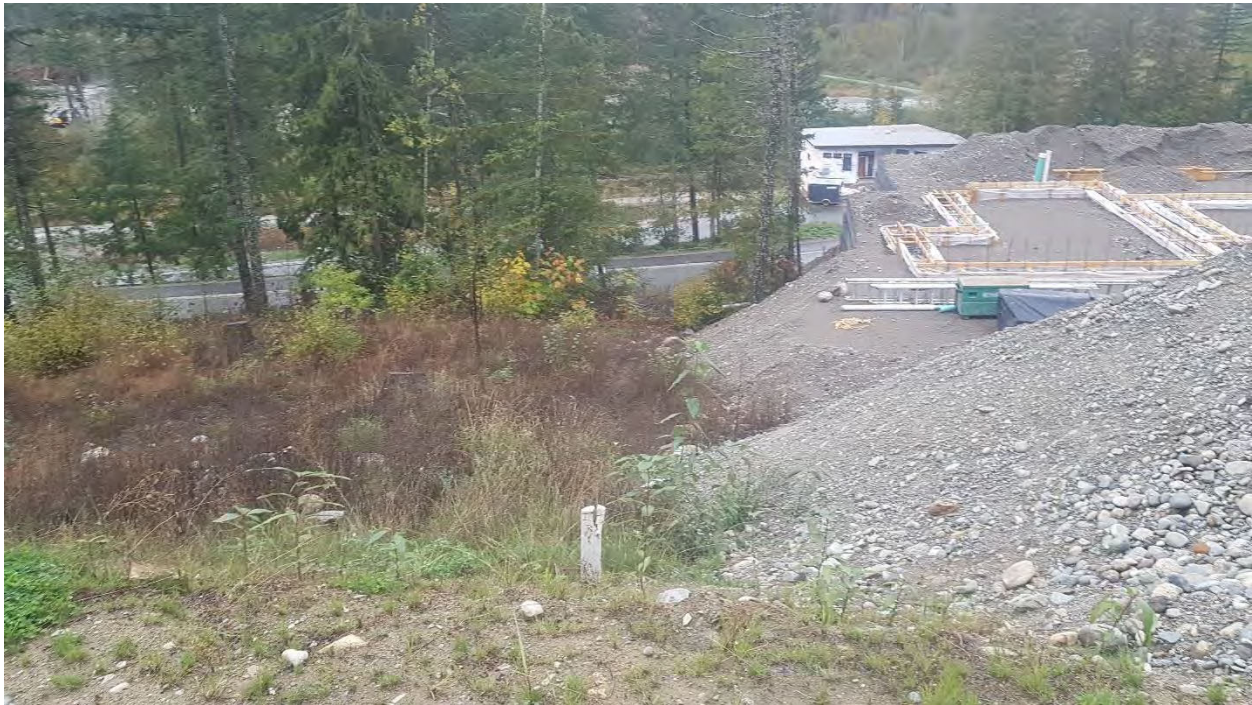
Photo D: Fill overflowing from # 7665 onto my lot
