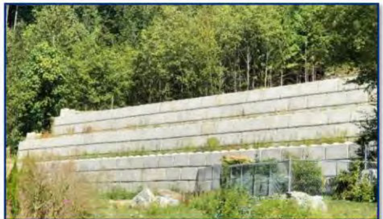
Unattractive visually dominant retaining wall.
