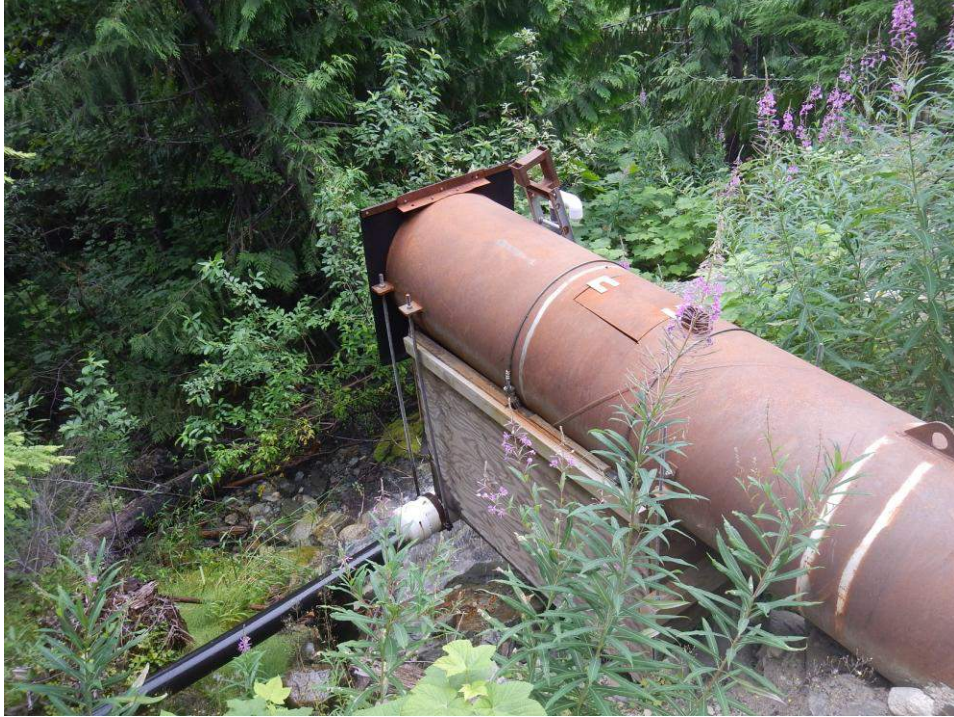
7.3 km water collection system for micro hydro system
