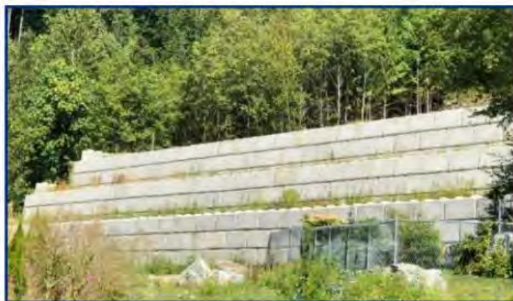
Unattractive visually dominant retaining wall.
