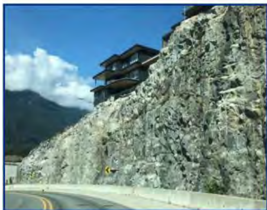
Blasted rock wall leaves stark and negative mark on the landscape.
