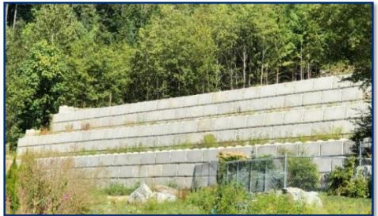
Unattractive visually dominant retaining wall.
