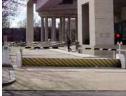
(Fig. 2.10) Pop-up barricades such as these are appearing more frequently due to security concerns. Unless security forces are constantly present to operate them, however, the fire department should be provided with a means to do so.
