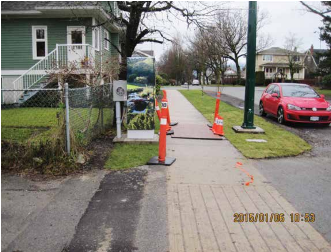
Close-up of connection cabinet
