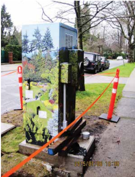
Close-up of connection cabinet
