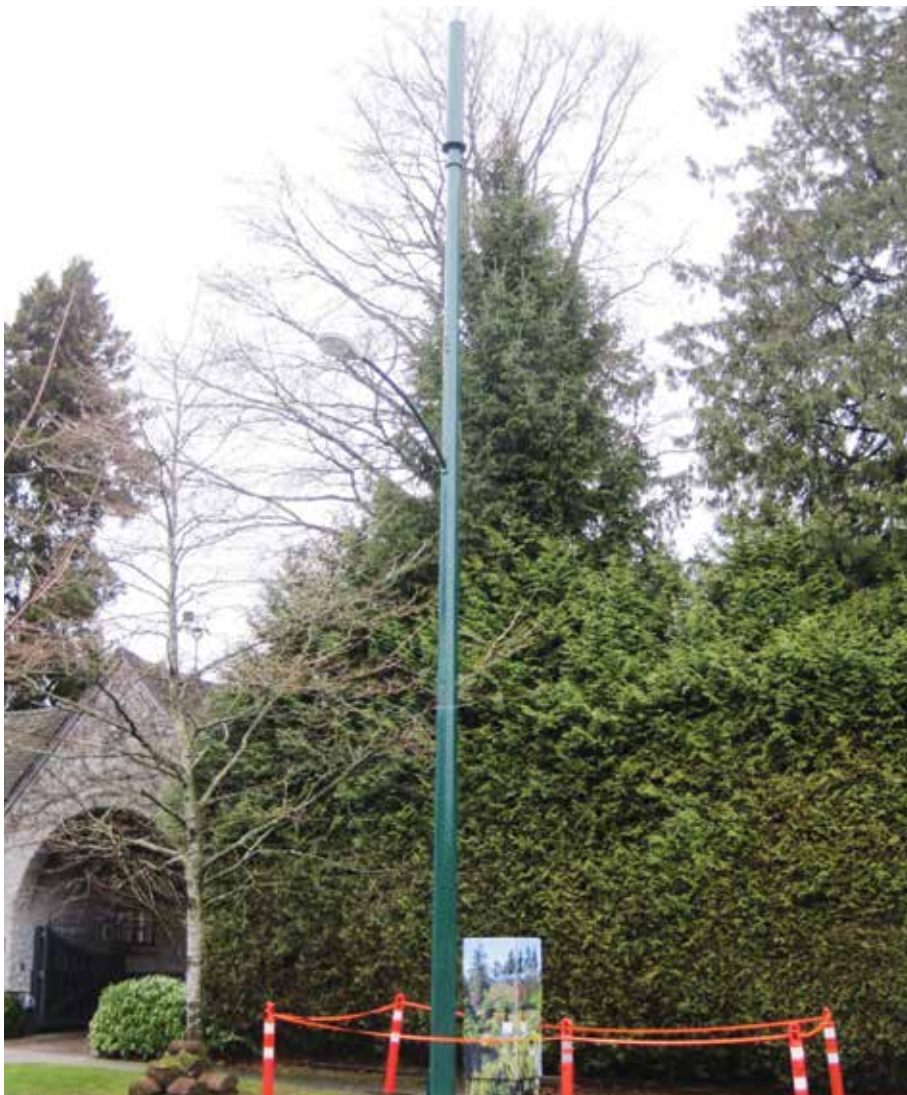
Example 1 of 13-metre tall streetlight antenna pole with connection cabinet at grade
