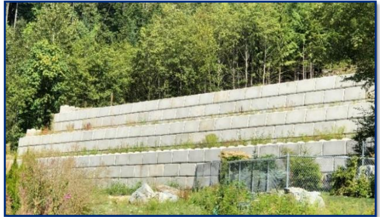
Unattractive visually dominant retaining wall.
