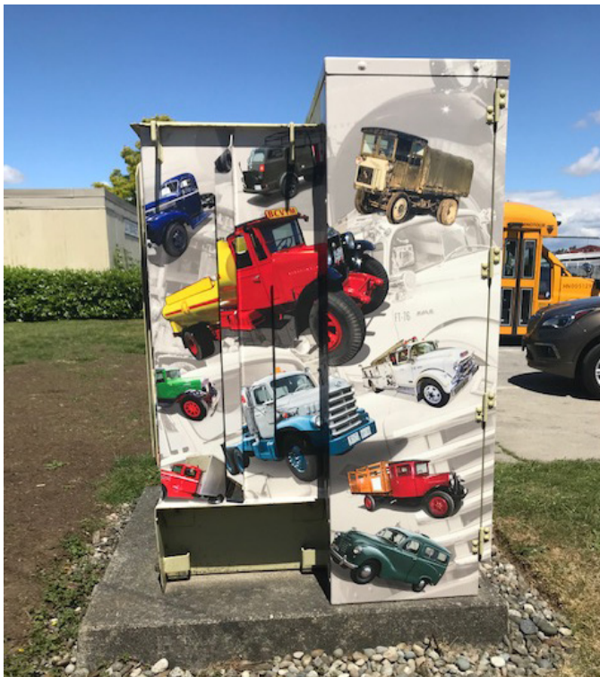
A wrapped pad-mounted transformer in Surrey.
