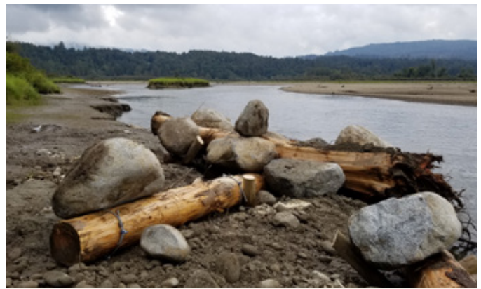
Floodplain restoration, using large wood and boulder structures, at Stave River. Photo credit: N. Cox.
