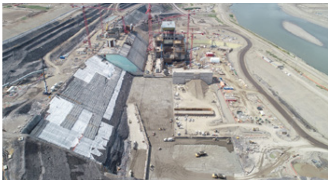
The Site C spillways excavation (foreground), powerhouse and main service bay, looking upstream, in July 2019.
