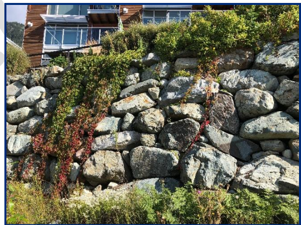
Retaining wall is made with natural building materials and visual impact minimized with natural landscaping.
