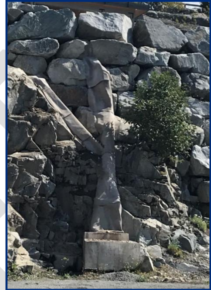
Visible utilities have a negative visual impact.
