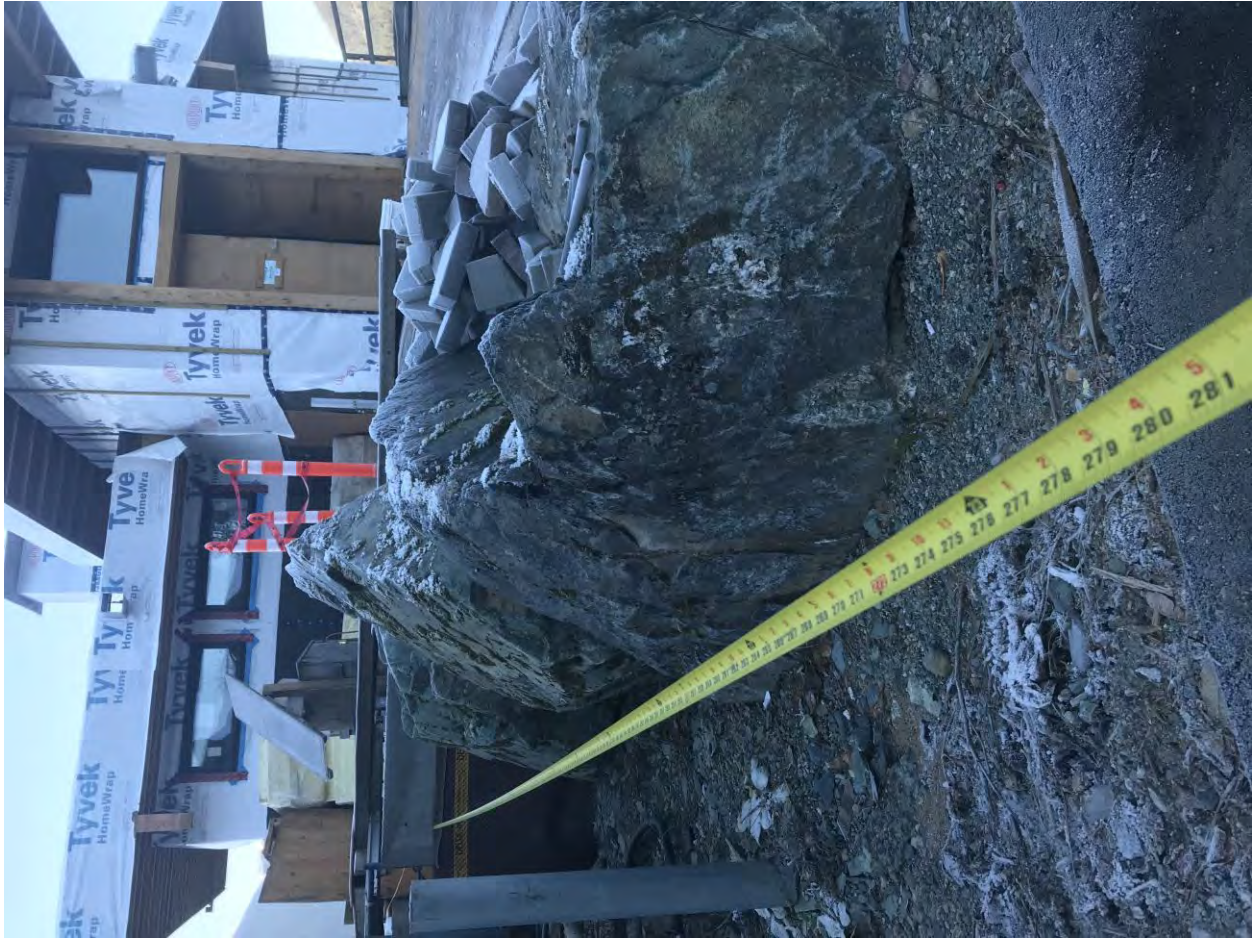
Building Inspection Photo – showing rock outcrop intruding into front setback (proof of hardship)
