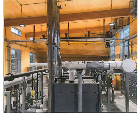
LMLGA -- Lower Mainland Local Government Association: City of Richmond for the Alexandra District Energy Building
