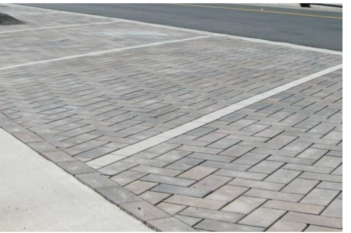
5 PERVIOUS PAVEMENT Permeable roadway pavers will be installed in strategic parking locations to reduce stormwater runoff.
