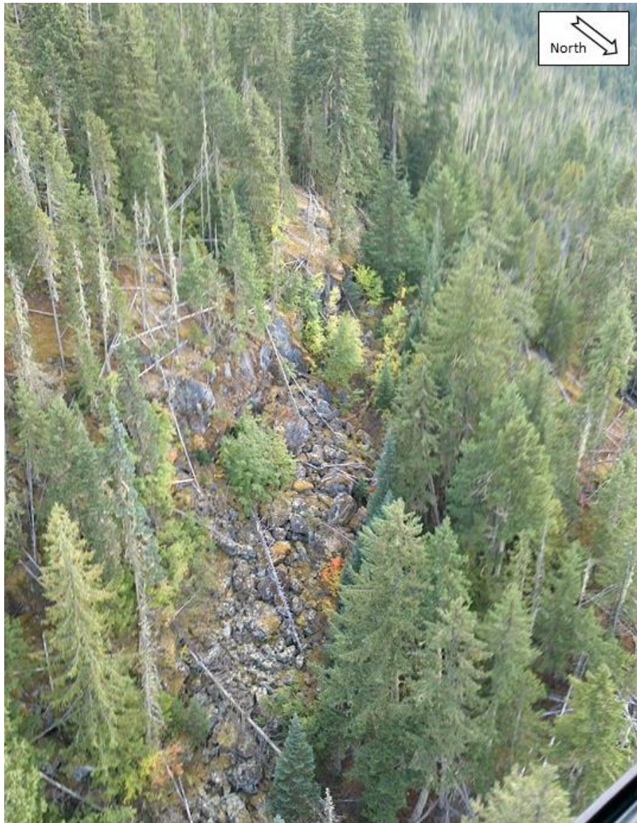
Photograph 23 Wide northeast trending tension crack filled with rock blocks and vegetation, and marking the upper limit of potential Source ID 13. The surface of the blocks is weathered and appears to be covered with lichen.
