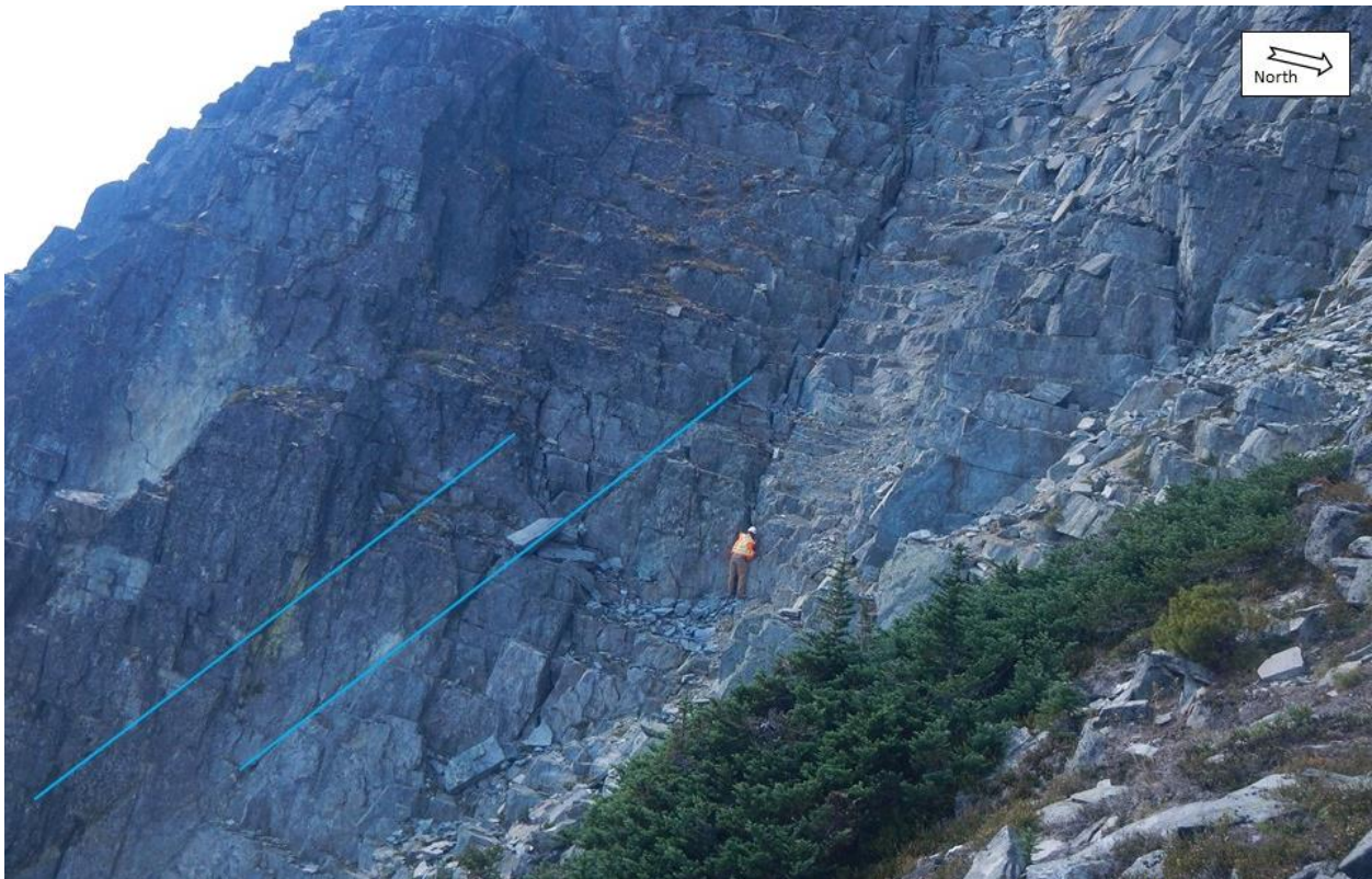
Photograph 2 D5 discontinuities on the southeast slopes, just downslope from the Mt Currie ridgeline.
