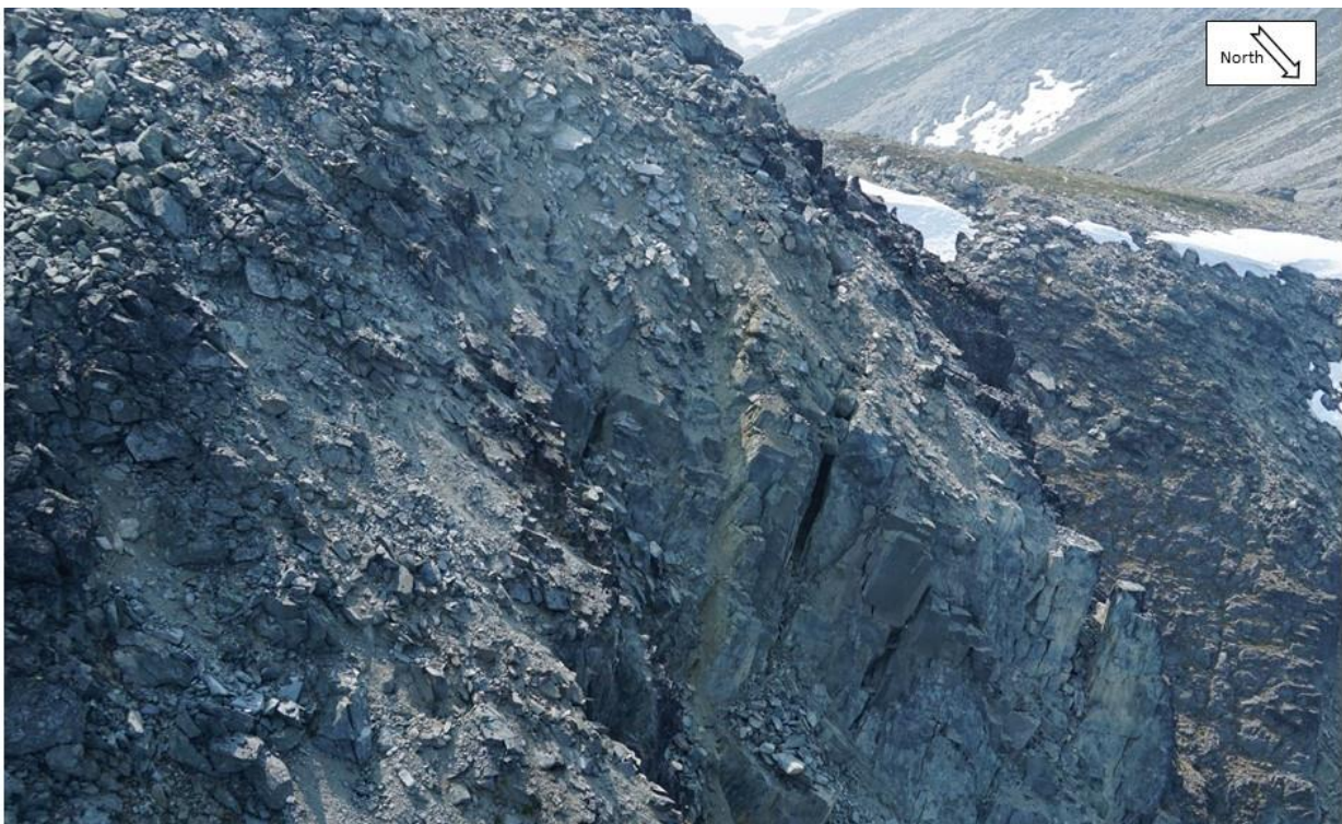
Photograph 30 Upper scar of rock fall event described in Photograph 28 showing dilation and open cracks corresponding to Source ID 7.
