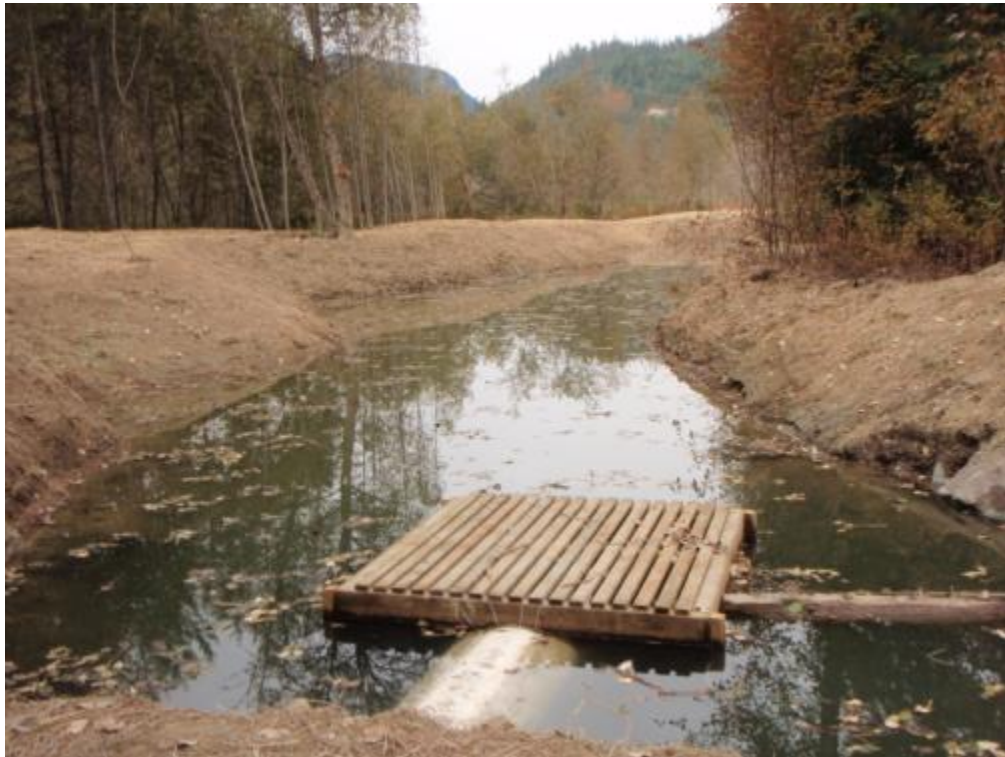
Figure 2. Beaver control installed in 2009 on culvert crossings at One Mile Lake Park.
