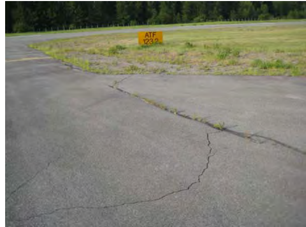
Traverse and random cracks on taxiway
