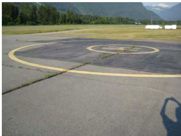
Cold joints on apron
