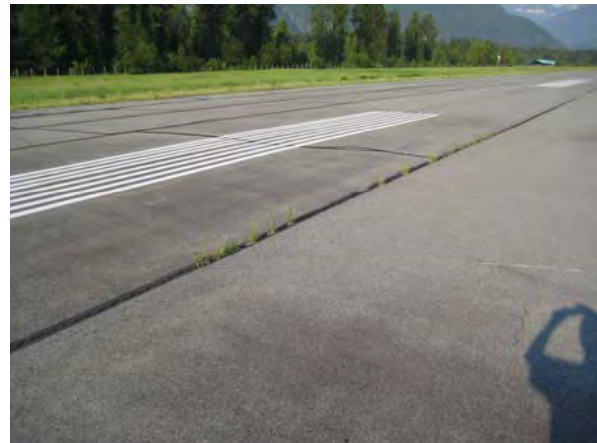
Cold joint crack running the length of the runway
