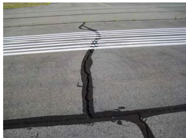
Traverse cracks on runway
