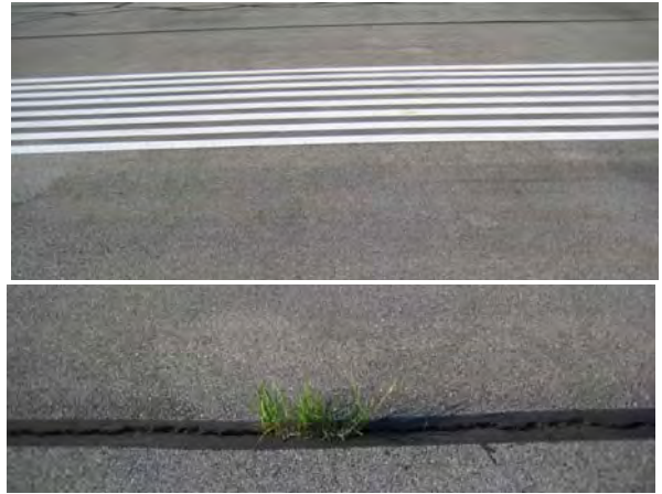
Cold joint on runway
