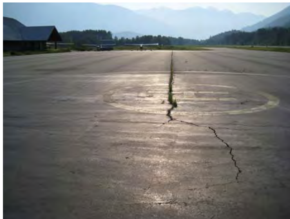
Cold joint cracks across the apron area
